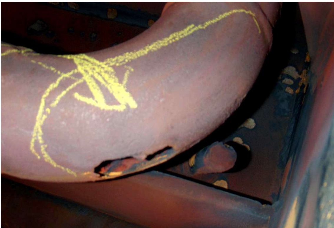
Figure 9 – Hole in Steam Supply Line in Condenser
