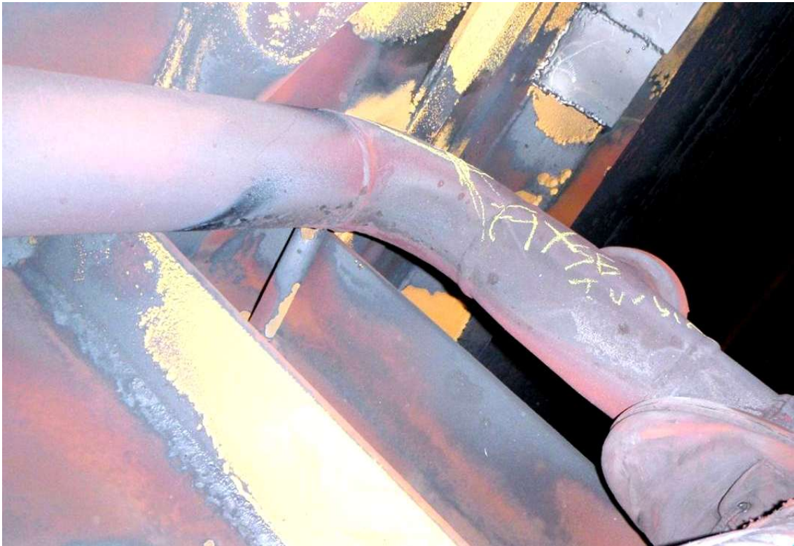
Figure 8 – Top View of Steam Supply Line in Condenser
