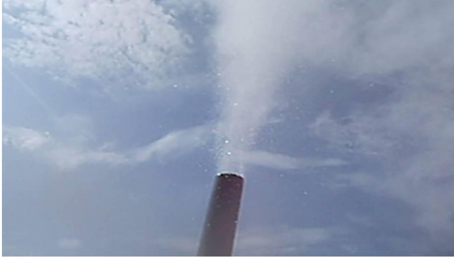
Figure 3: Example of Moderate Water Entrainment in Deaerator Vent
