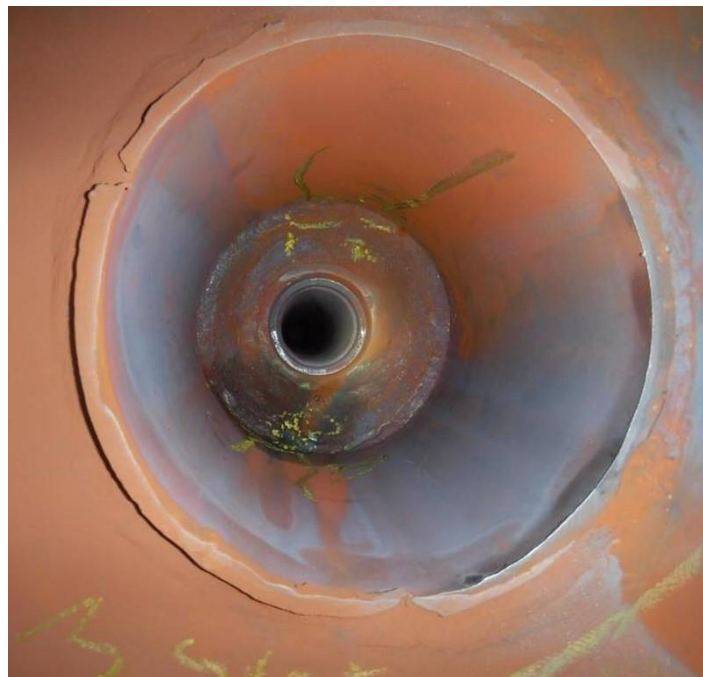
Figure 6: Example of Water Spraying From Water Inlet Chest Into Vent Offtakes
