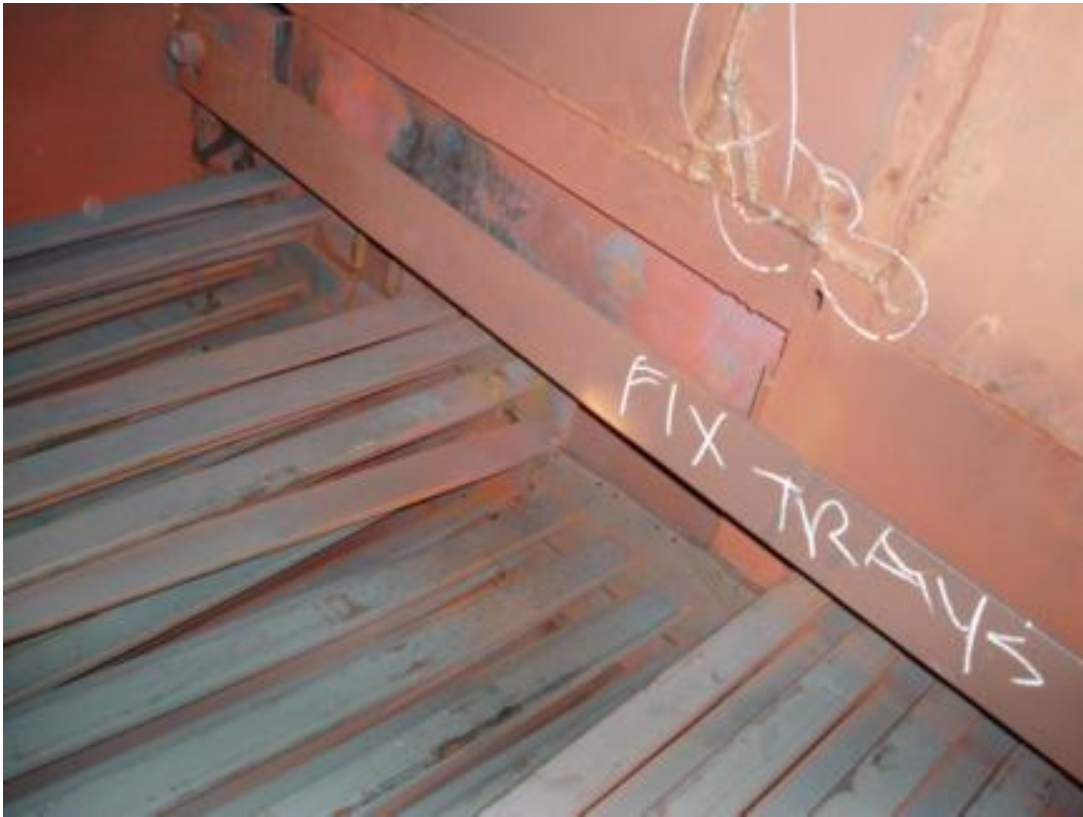
Figure 17: Complete Bundle Removal Required
