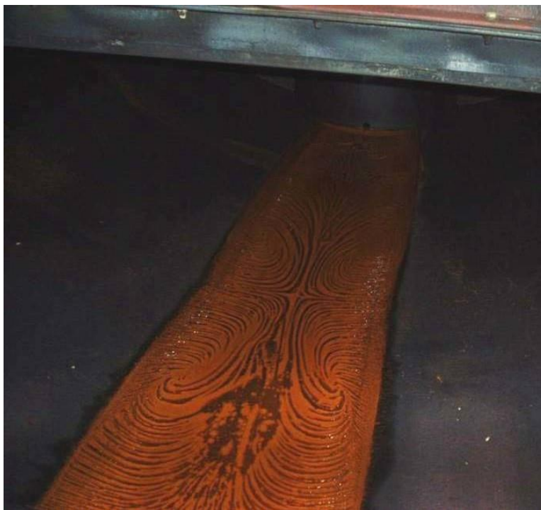
Figure 18: Erosion of Deaerator Floor
