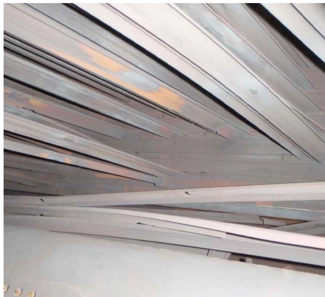
Figure 15: Failed Single Trays
