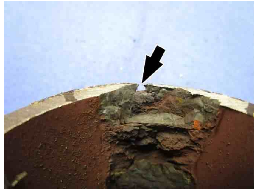
Cut through point of failure prior to mounting
